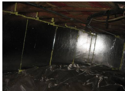
Figure 2151-1: Foil-faced rigid foam board on foundation walls, vents sealed and continuous and sealed
