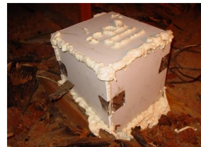
Figure 2131-1: Recessed light covered with drywall box
