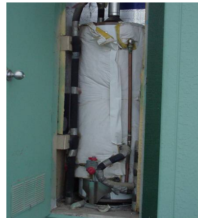
Figure 412-1: Existing mobile home water heater
