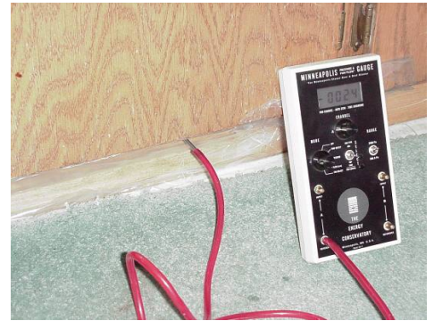
Figure 1141-1: Toe-kick sealed with duct mask tape; pressure pan reading of 24 Pa!
