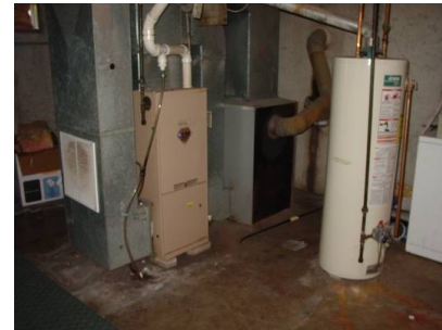
Figure 312-2: Combustion appliance zone: note presence of grille in return air duct that can cause depressurization of the water heater
