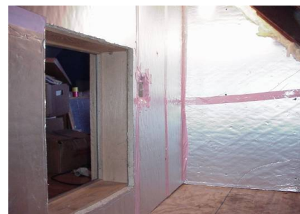
Figure 21364-2: Fiberglass insulation covered with foam board used as an air barrier
