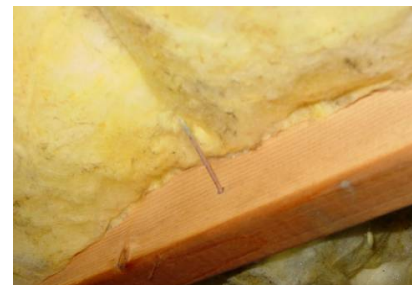
Figure 2152-3: Compressed insulation due to insulation support
