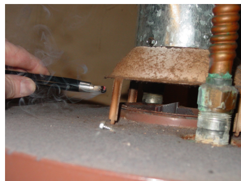
Figure 117-2: Failed spillage test
