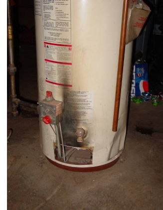
Figure 31111-1: Evidence of flame roll-out
