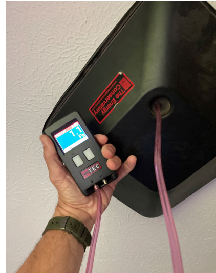
Figure 1142-1: Tight duct measuring 1.1 Pa
