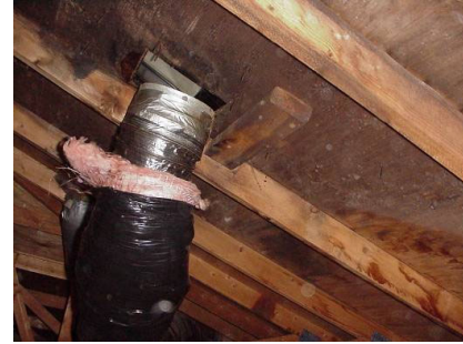
Figure 507-2: Venting to a roof vent is not allowed under the Weatherization Program; a roof vent may be removed and the exhaust duct extended through the existing hole and capped with a termination kit
