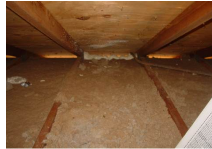
Figure 2122-13: Exterior wall top plate under low-pitch roof sealed with foam gun shown in Figure 2122-10.
