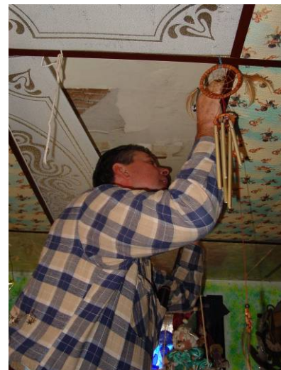
Figure 1111-2: Remove a ceiling tile to relieve pressure
