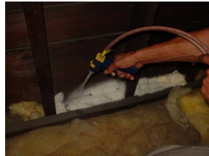
Figure 2122-4: Study cavity blocked with batt insulation and sealed with 2-part spray foam
