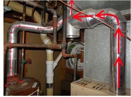
Figure 312-3: Checking for spillage at the water heater after firing the furnace
