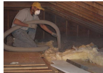
Figure 21331-1: Required attic insulation R-value is a minimum of 49 or the maximum amount with an SIR greater than 1.0
