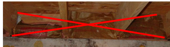
Figure 217-1: Batt insulation is not permitted to be used for rim insulation
