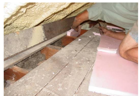
Figure 21364-4: Connecting roof thermal boundary to sidewall thermal boundary with rigid foam board insulation; 2-part spray foam will also work
