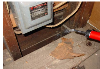
Figure 2121-1: Smoke being drawn down an open study cavity indicating leakage to the inside
