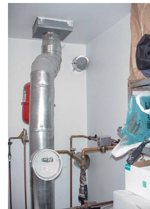
Figure 3124-2: Combustion air intake
