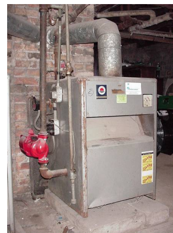
Figure 3161-1: Warm water boiler
