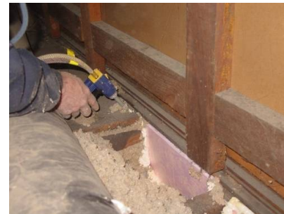
Figure 2122-1: Sealing joist cavity under knee wall with foam board and 2-part spray foam
