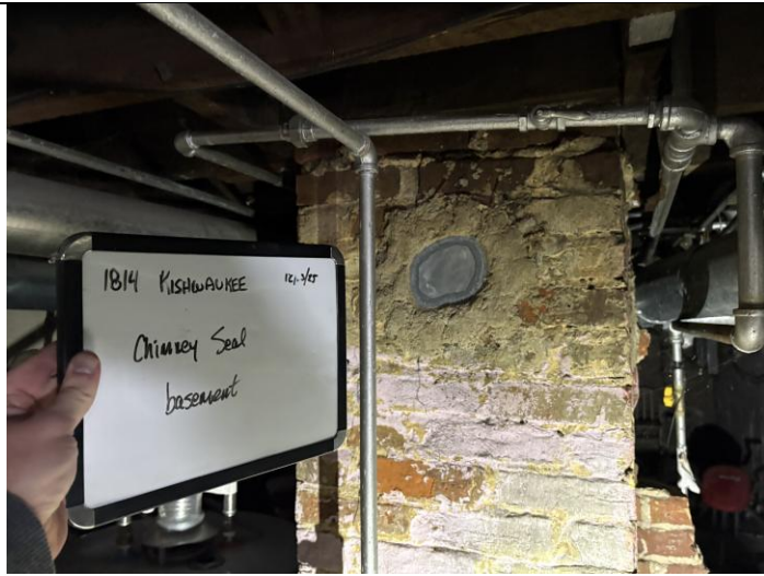
Date: 12/10/25 Location: Basement Description: Chimney Seal
